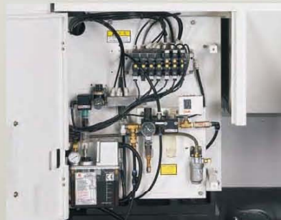
Hydraulic & Lubrication System(LU-620)
