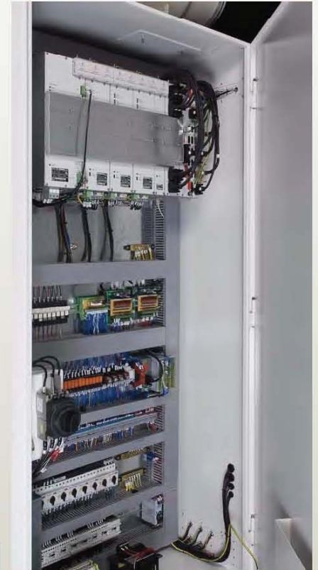
Electric System For Easy Maintenance
